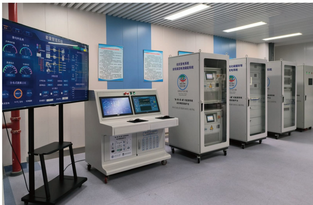
图7 (网络版彩色)“源-网-荷-储”式异质能流复合供能系统动态调控实验平台原理图及实物图 Figure 7 (Color online) Schematic diagram and physical diagram of the dynamic experimental platform of the generation-grid-load-storage type integrated system with heterogeneous energy flows
